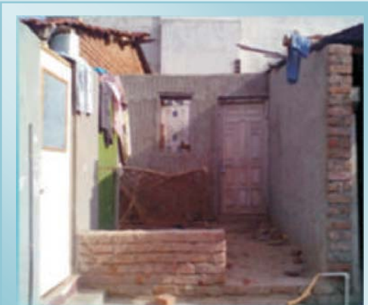
Picture-1: IAY house in Moraj village in Tarapur taluka of Anand district
