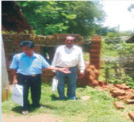
IAY house in scheme No. 115/2010-11 at Forest Block GP in Gurabanda block of East Singhbhum district abandoned after ₹ 48,500 (final payment) was paid to the beneficiary.
