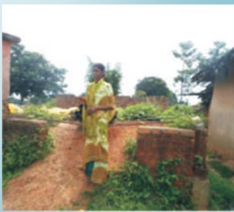
IAY house in scheme No. 67/2009-10 at Pali GP in Ratu block of Ranchi district abandoned after ₹ 35,000 (final payment) was paid to the beneficiary.
