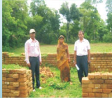
IAY house in scheme No. 115/2010-11 at Forest Block GP in Gurabanda block of East Singhbhum district abandoned after ₹ 48,500 (final payment) was paid to the beneficiary.
